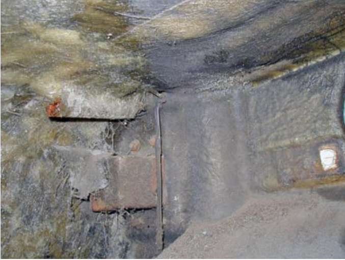
The body inside the wings should be fairly smooth. Rough fibreglass work like this indicates past damage that has been repaired.
